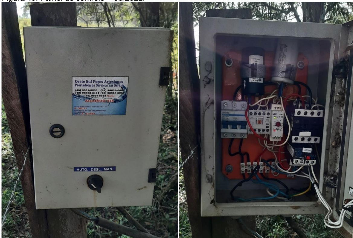
Figura 40: Paineis de controle – 06/2021.
